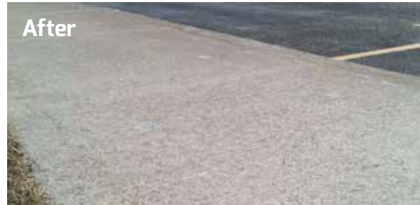
After ■ The stabilizing grout mixture helps to raise the slabs, and the holes are then patched to complete the project.
