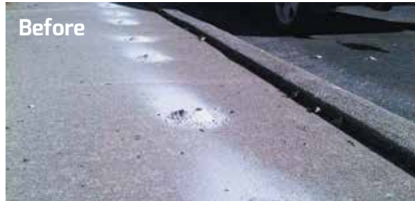
Before ■ Sidewalk before raising. Holes were drilled through the sunken slabs and a stabilizing mixture was pumped under the slabs.
